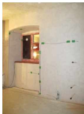
Figure 12: The testing of the insulating mortar ISOCAL at the case study in Benediktbeuern
