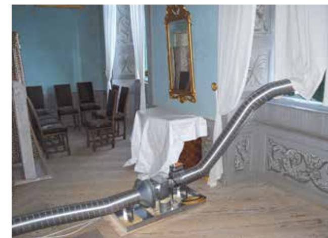
Experimental setup for indoor climate control using adaptive ventilation at Skokloster Castle, Sweden (Figure 2b)
