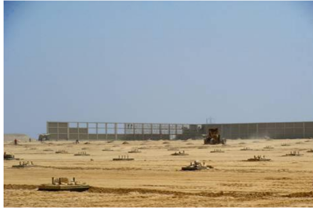
Figure 16 Construction site of parabolic trough solar field at Kuraymat (Egypt) with the foundations of the solar field
